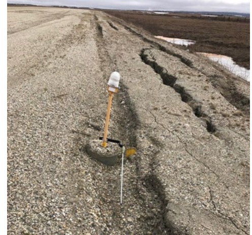
Figure 4. Shoulder Rolling Interfering With the Lighting System at Noorvik Airport (D76) [DOT&PF, 2019].
