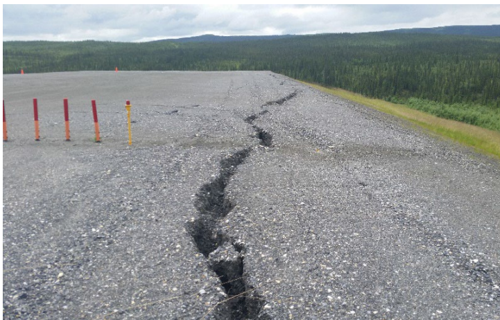
Figure 6. Longitudinal Cracking at Kiana Airport (IAN) [DOT&PF, 2023].
