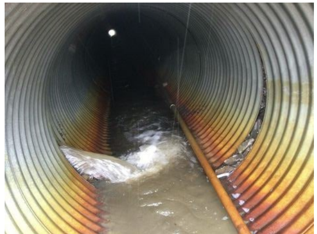
Figure 10. Takotna (TCT) Runway Cross Culvert Failure Caused by Differential Settlement.
