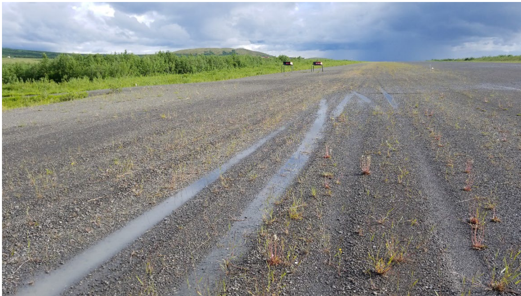
Figure 9. Rutting of the Runway Surface at St. Mary's (KSM) (Photograph taken by DOT&PF, 2021).
