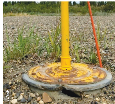
Damage to edge light base, likely from snow plowing.
