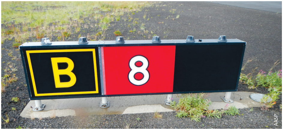
Airports with multiple runways feature lighted runway and taxiway signs to guide pilots, like this one in Unalakleet.
