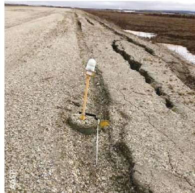
Damage can occur due to embankment failures, settlement, erosion, and permafrost thaw, as seen here with a runway edge light in Noorvik.
