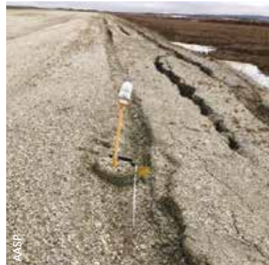
Damage can occur due to embankment failures, settlement, erosion, and permafrost thaw, as seen here with a runway edge light in Noorvik.
