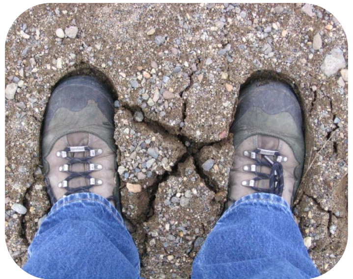
Soft runway surface at South Naknek Airport
