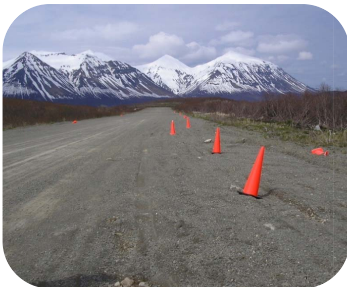
Rutted runway at Chignik Lake Airport – cones have been placed to mark the areas of deepest rutting
